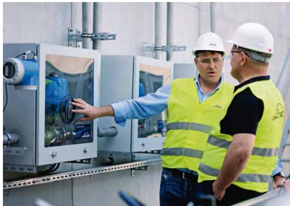
Darren Gurney, Senior Process & Business Development Manager (left), and Omer Saray, Applications Engineer (right), go over the details of the CO 2 dosing system.
